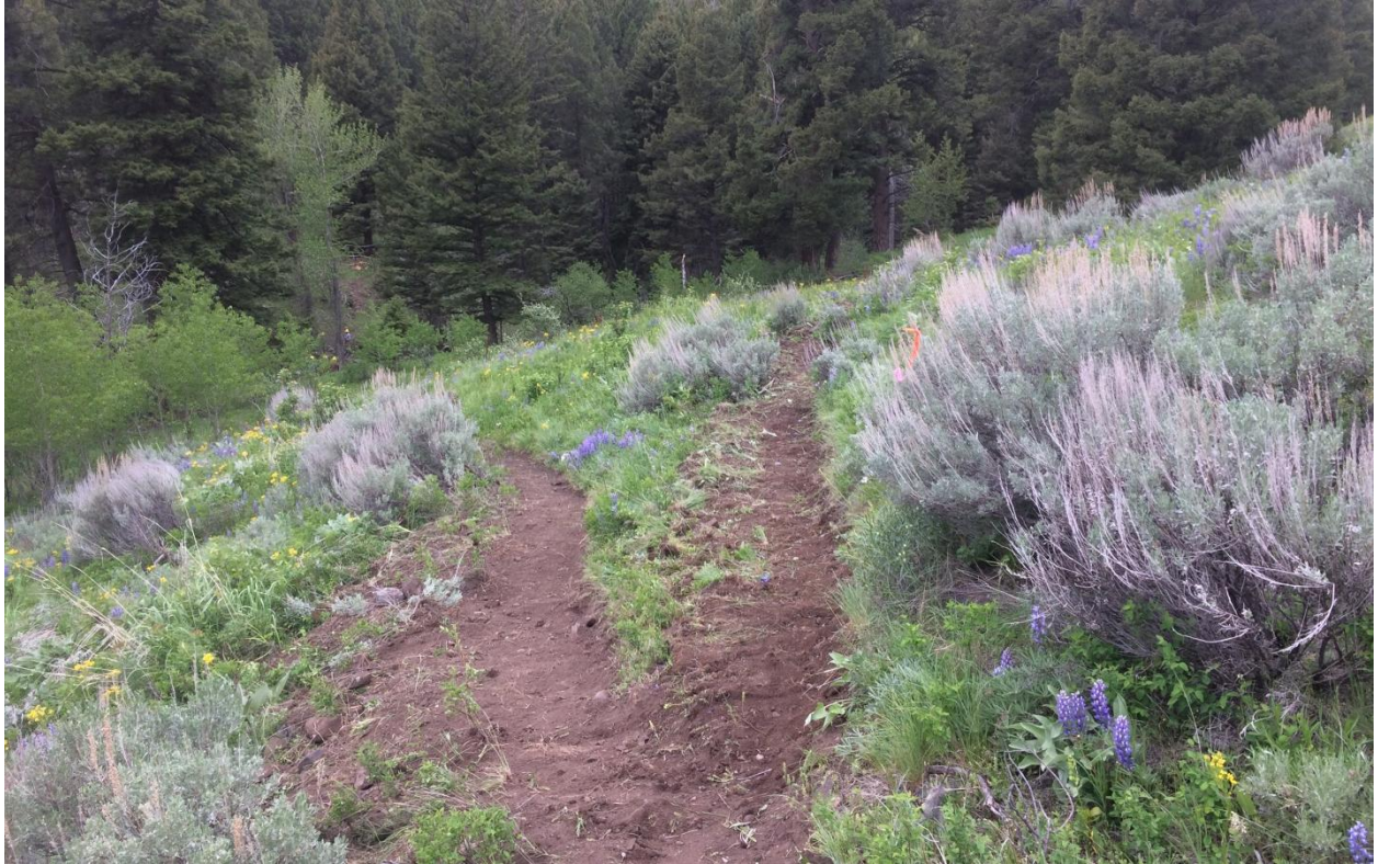
YEP Volunteers recreated a tread 50 yards long that connects the upper Williams Creek Trail to the Lower Williams Creek Trail. This continuity had been lost in the sage brush and an abandoned range fence. (Above and below photos)
